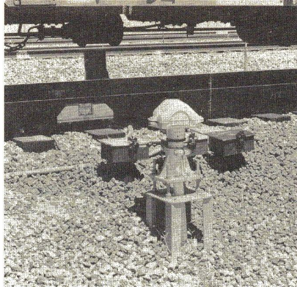
Servo Hot-Wheel Scanner installed at Wayside Detection Research Facility. Diagonal line of sight of infrared scanner scans four wheels of passing truck in turn, obtains ambient-temperature reference from stationary target on opposite side of track between wheel intercepts.
